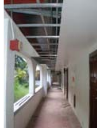
Corridor chase opening for A/C.
