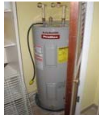
Hot water heater electrical ready.
