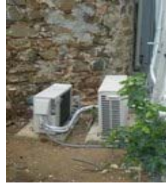
A/C condensers installed.
